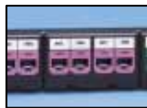
Patch panel labels
