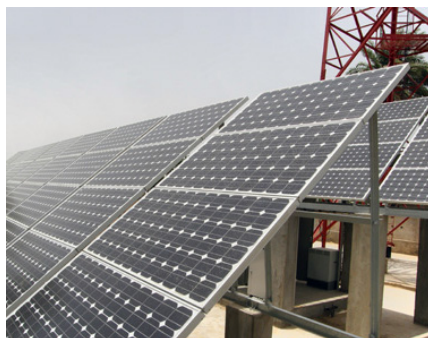
Solar-powered Cellular Base Station
