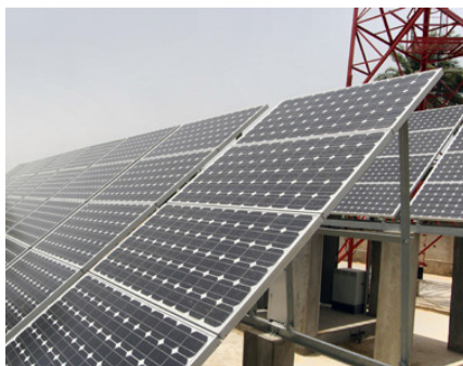
Solar-powered Cellular Base Station
