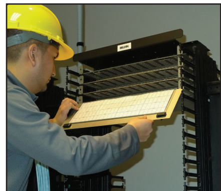
Shelf identification labeling is clearly visible.
