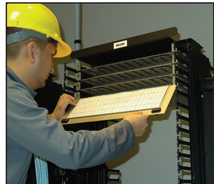
Shelf identification labeling is clearly visible.
