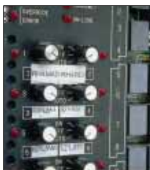
Label switches, relays and other devices
