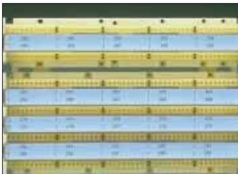
Network Systems Labeling
