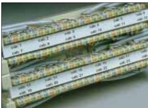
Network Systems Labeling
