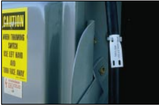
Identify wires, cables or equipment requiring removable and reusable information
