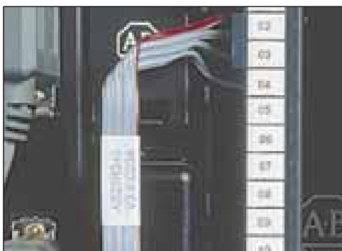
Terminal Block Labeling
