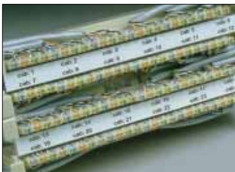
Network Systems Labeling
