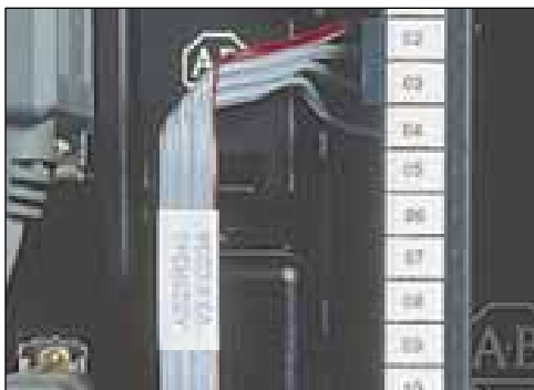
Terminal Block Labeling
