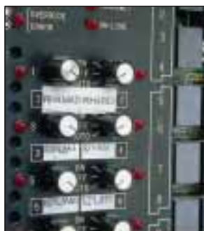
Label switches, relays and other devices
