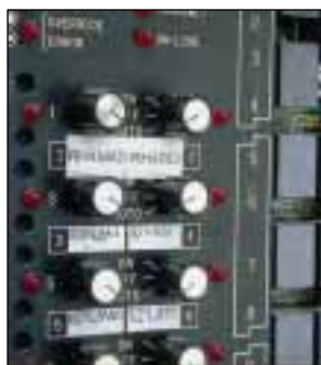
Label switches, relays and other devices
