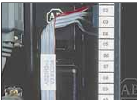
Terminal Block Labeling
