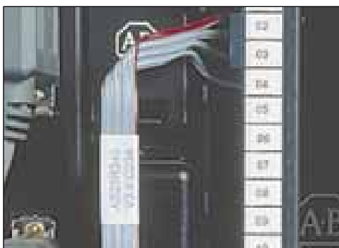
Terminal Block Labeling
