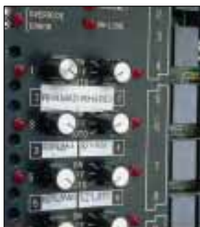
Label switches, relays and other devices
