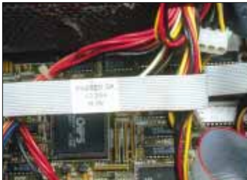
Flat Ribbon Cable Labeling
