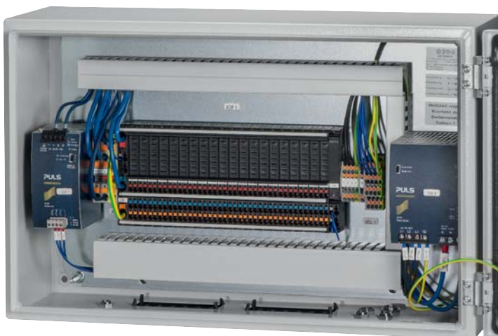
Decentralised power distribution unit DC 24 V
