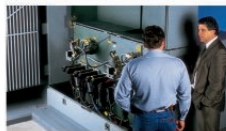
COOPER Power Systems
