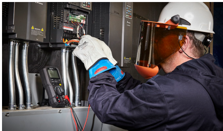
Troubleshoot Variable Frequency Drives using VFD mode
