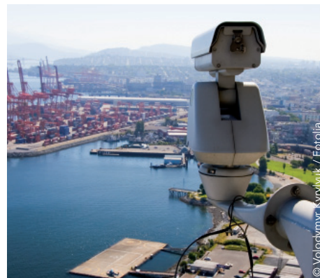
Building Automation & Control
