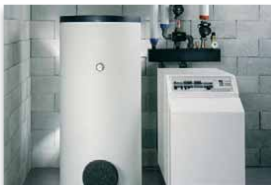
■ Control of heating and hot water system: Heat pump
