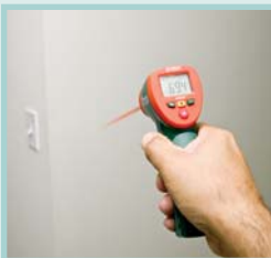
Check building for insufficient insulation
