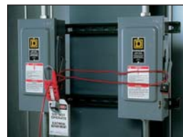
Lockout single or multiple electrical disconnects
