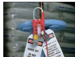
Lockout gate valves
