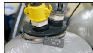
General Mechanical Identification
