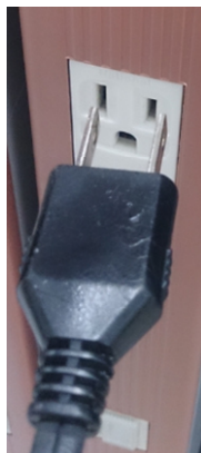
Figure3. Power outlet connection
