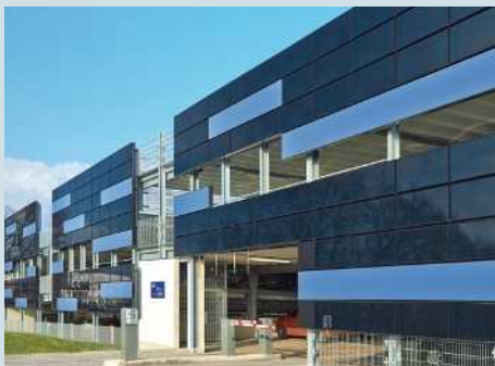
Building-integrated photovoltaics (BIPV)
