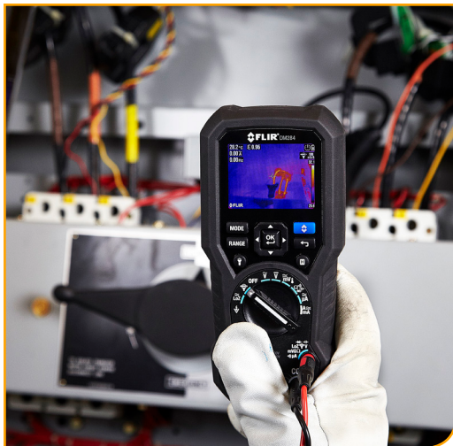
Thermal scan of an electrical panel
